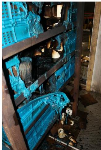
Figure 3-25: Post-test image of damage to the vented ML-ASRS containers and the internal corrugated boxes.
