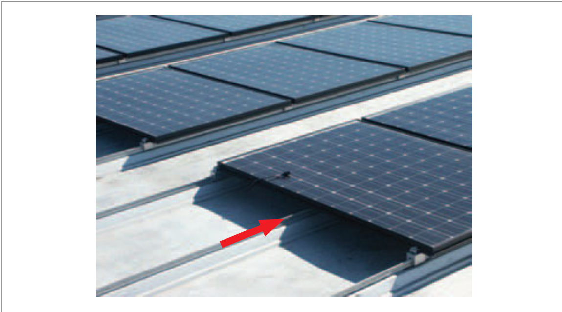
Fig. 3.4.5-2. Unacceptable arrangement unless specifically tested and FM Approved: clamp missing from SSR rib below middle of outer panel edge
