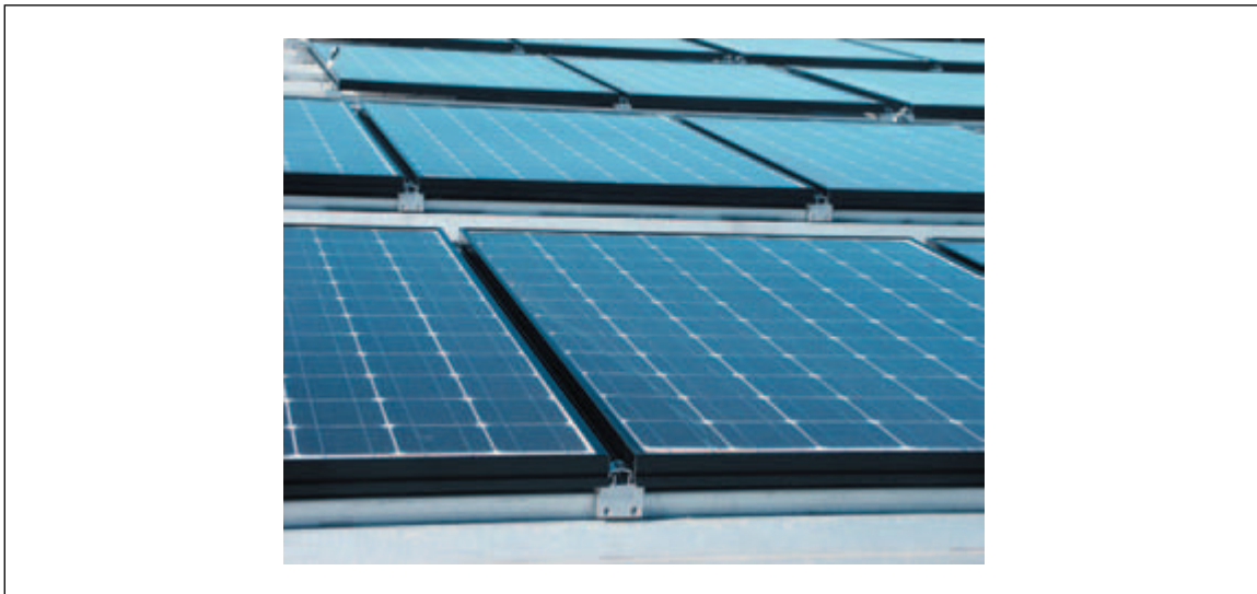
Fig. 3.4.5-1. Solar panels secured to standing seam roofs using external seam clamps
