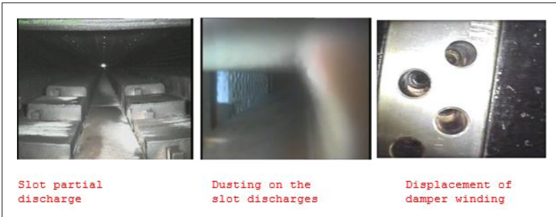
Fig. 2. Examples of footage taken during robotic inspection (Photo by courtesy of 3angles, Inc. and Iris Power)
