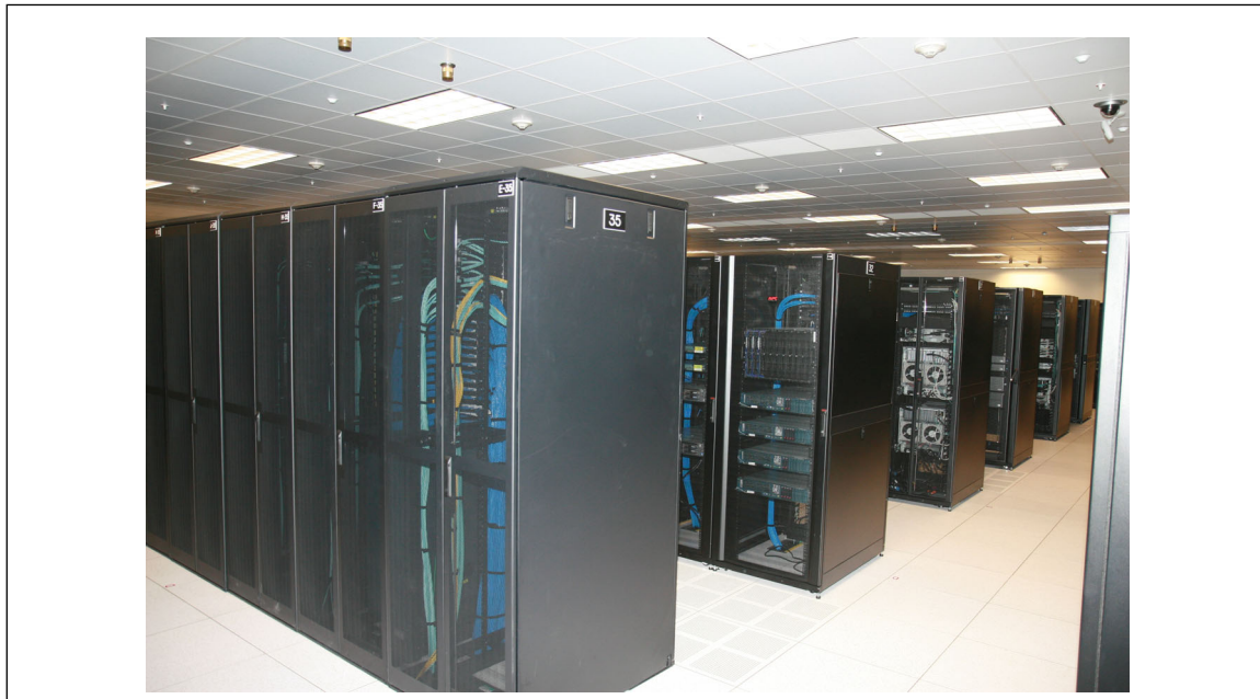
Fig. 2.3.2.5.2. Typical server cabinet and rack arrangement
