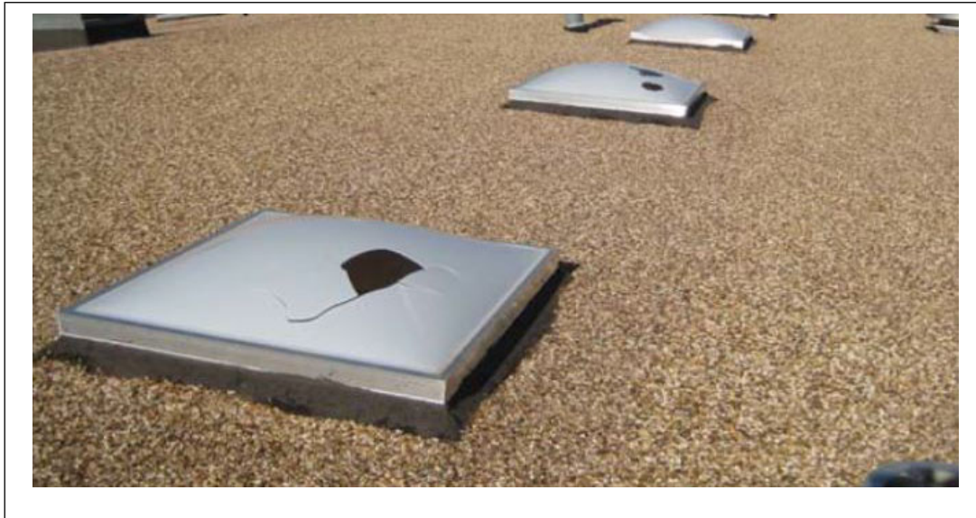
Fig. 3.2.1-1. Holes in acrylic skylights caused by hail
