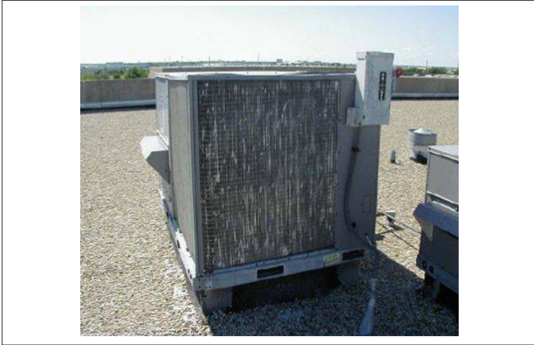
Fig. 3.3.1-1. Hail damaged HVAC unit
