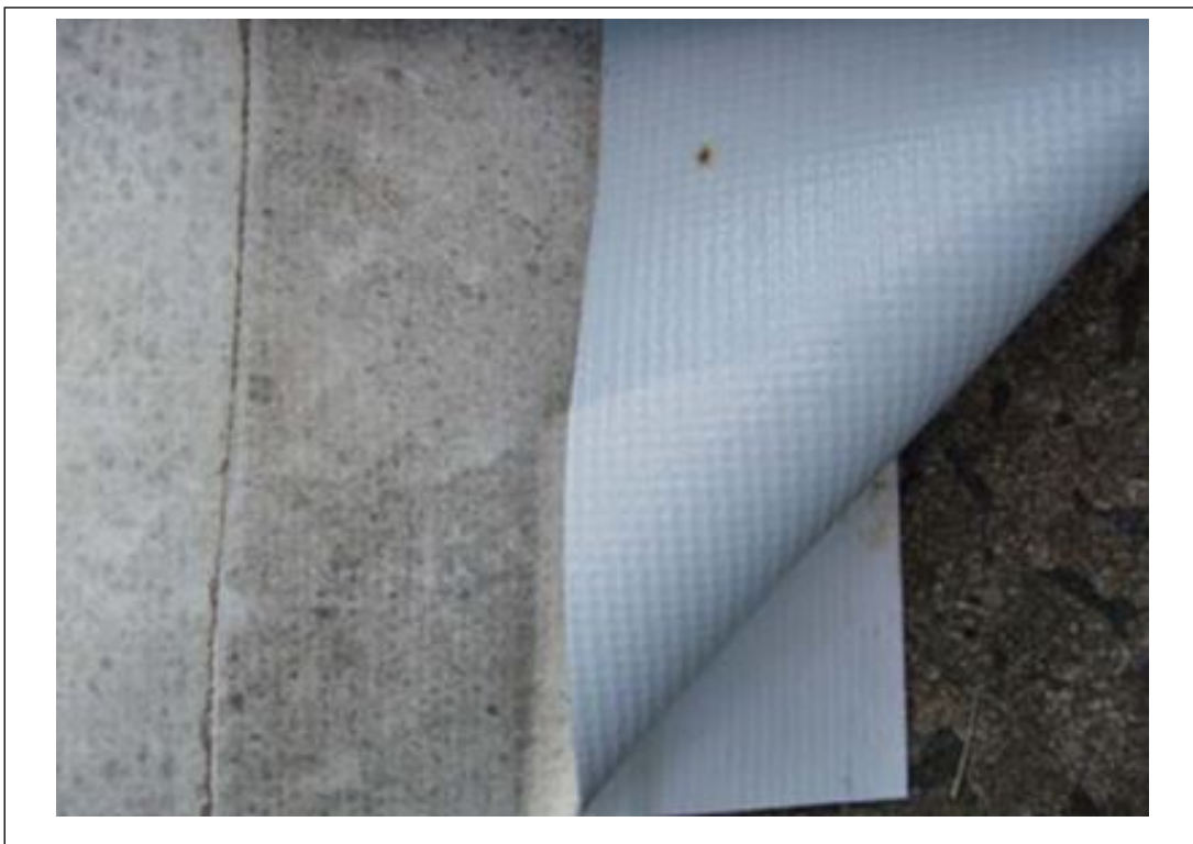
Fig. 3.5.2-4. Roof cut from hail-damaged roof in Figures 3.5.2-1 and 3.5.2-2
