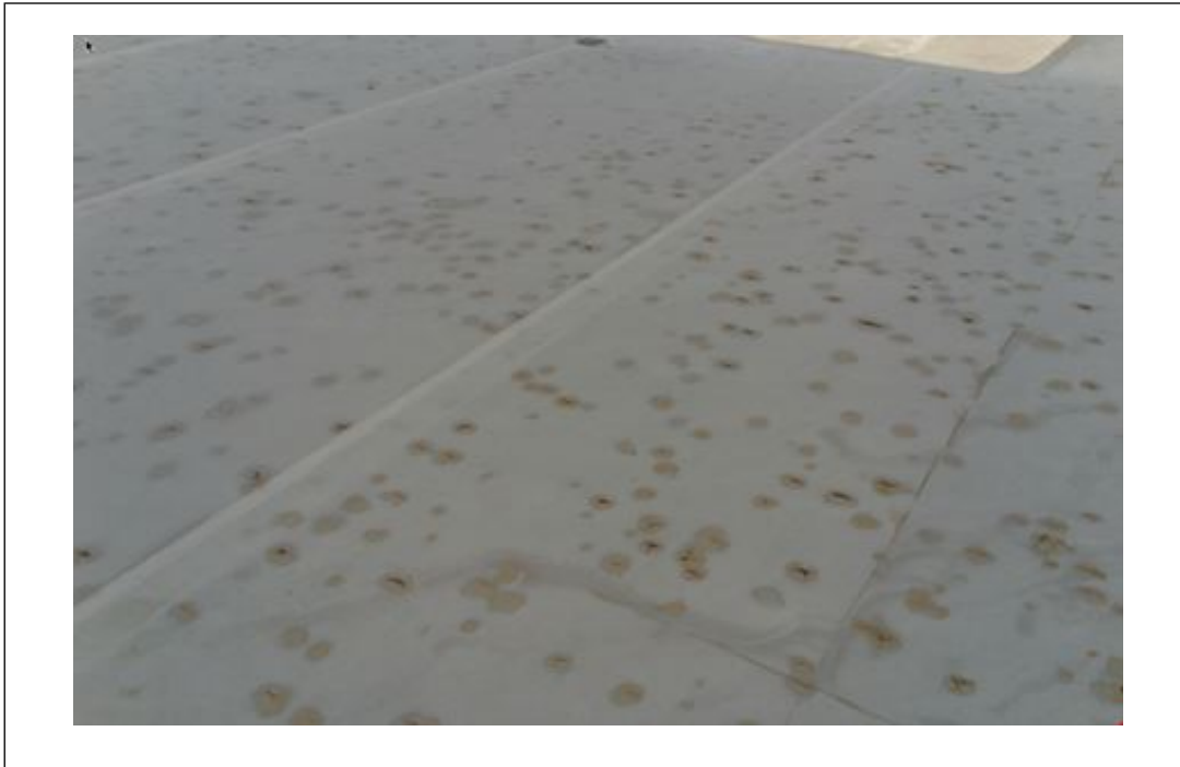
Fig. 3.1.1-1. Single-ply membrane roof 0.045 in. (1.1 mm) thick cut by hail
