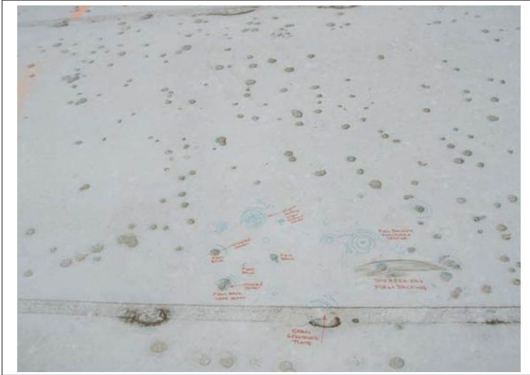
Fig. 3.5.2-1. Hail damage to 15-year old single-ply membrane
