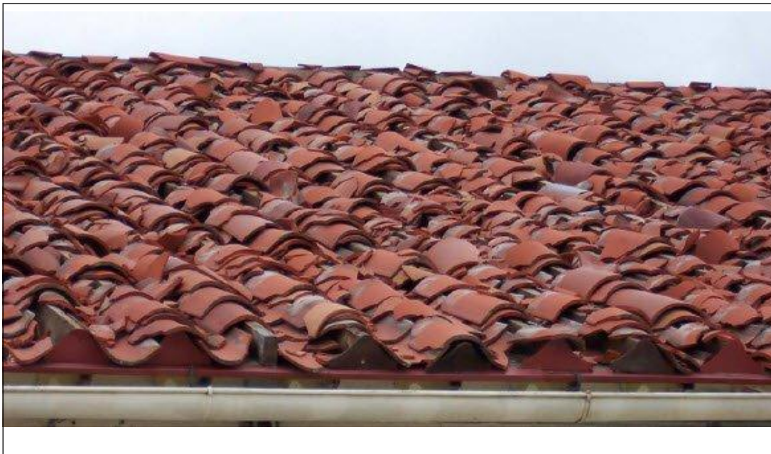
Fig. 3.8-2. Hail damage to clay roof tiles
