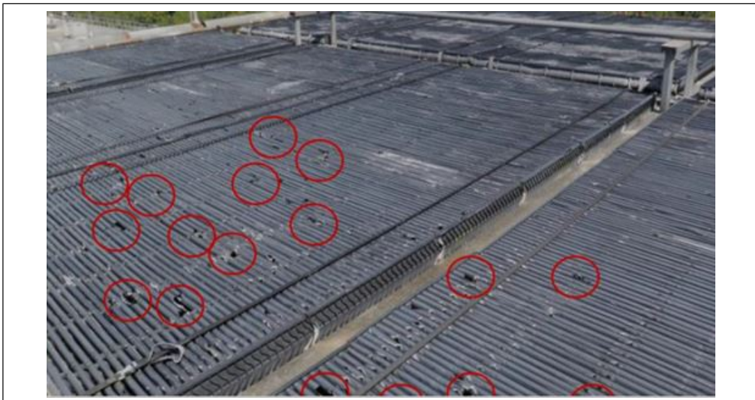
Fig. 3.4.1-2. Hail damage to plastic drift eliminators
