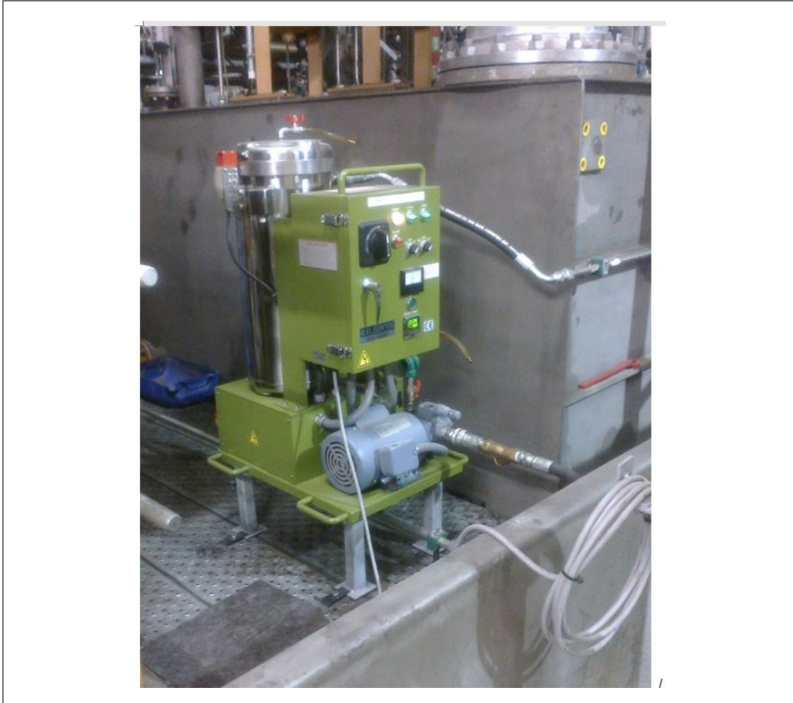
Fig. 2.2.5.4.1. Lube oil purifying skid inside containment area
