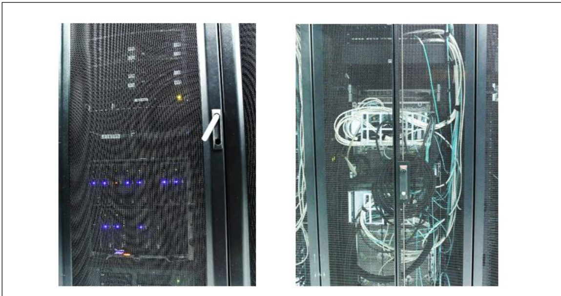
Fig. 1. Front and rear of server racks with locks
