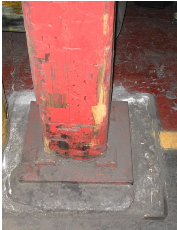
Fig. 3.1-5. Base of unanchored building column resting on floor
