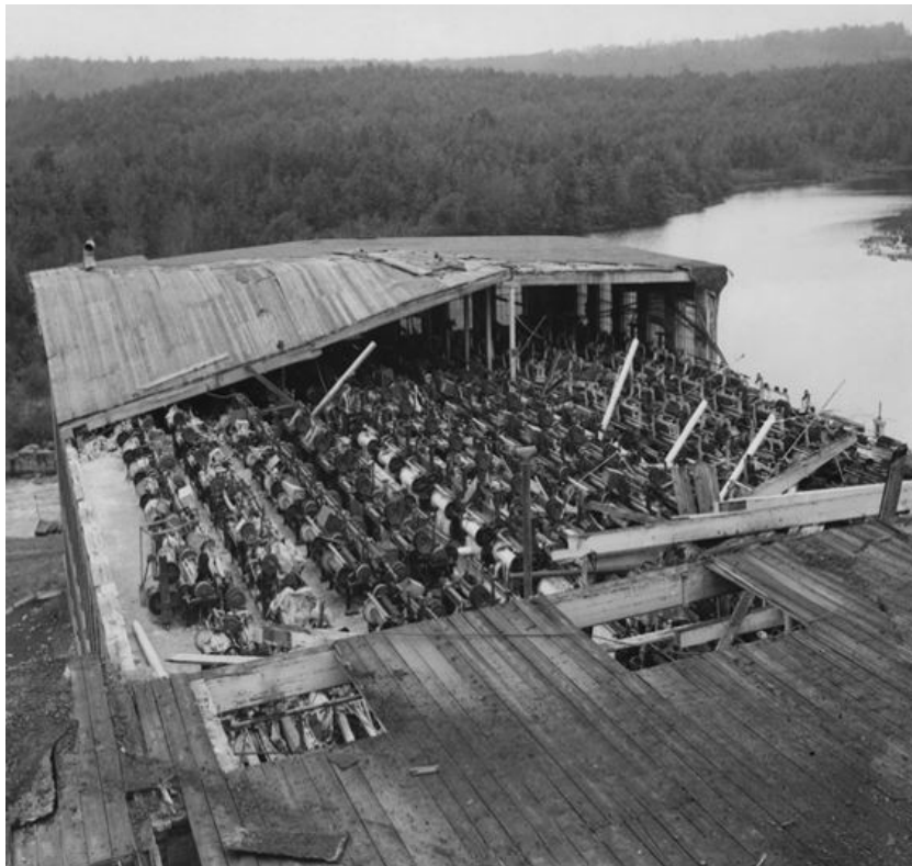
Fig. 1.1-1. Roof damaged in the 1938 New England Hurricane (after debris removal)
