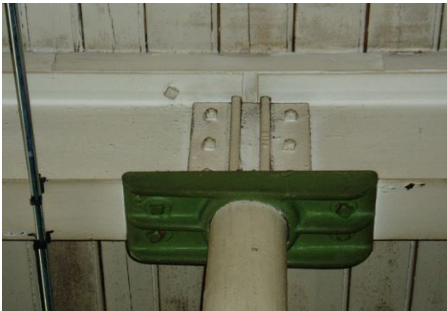
Fig. 3.1-3. Closeup of column cap (green) in Figure 1.1-3 (the column cap is not secured to the column)
