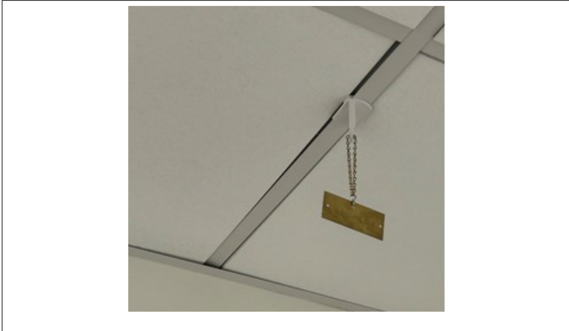
Fig. 2.4.2-2. Brass label showing water shutoff valve above drop ceiling
