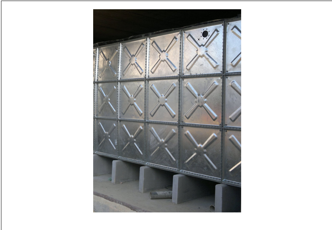
Fig. 2. Pressed steel suction tank
