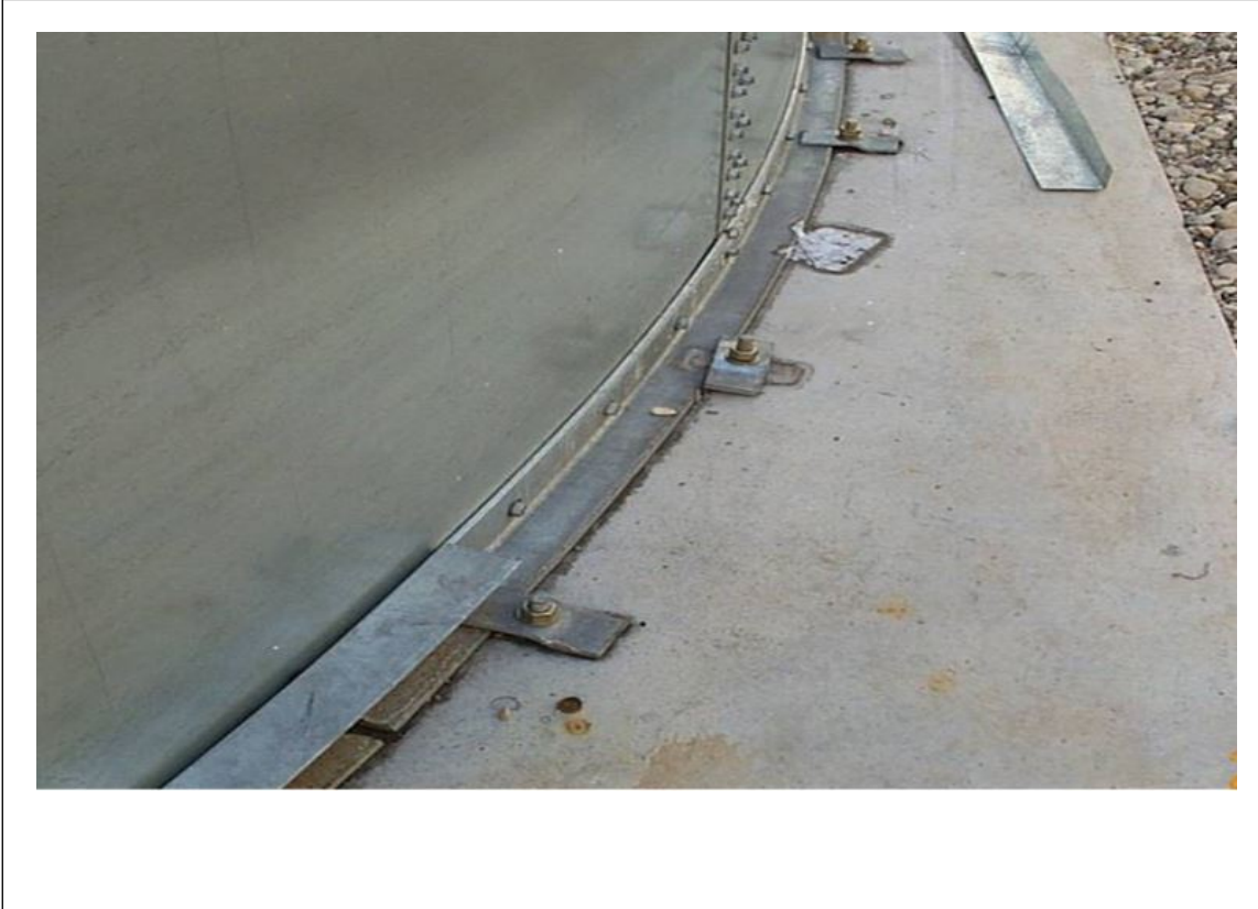
Fig. 29. Inadequate suction tank anchorage
