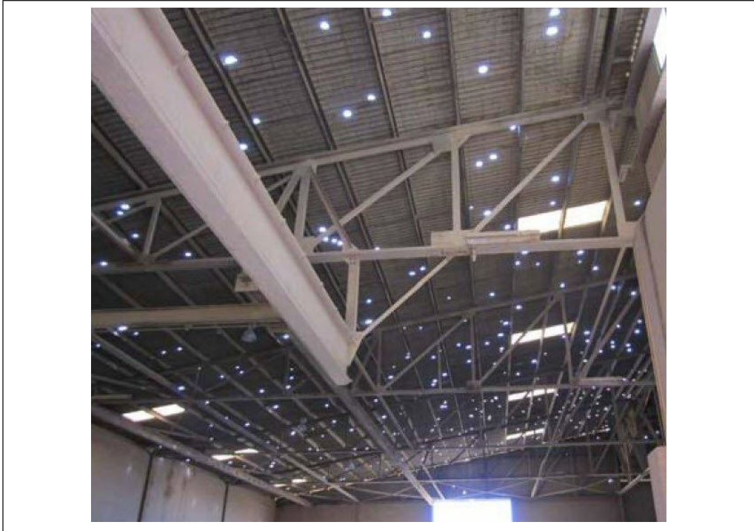
Fig. 3.8-1. Hail damage to asbestos cement roof
