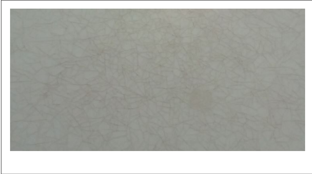
Fig. 3.2.1-3. Close up of embrittled acrylic skylight in Fig. 3.2.1-2
