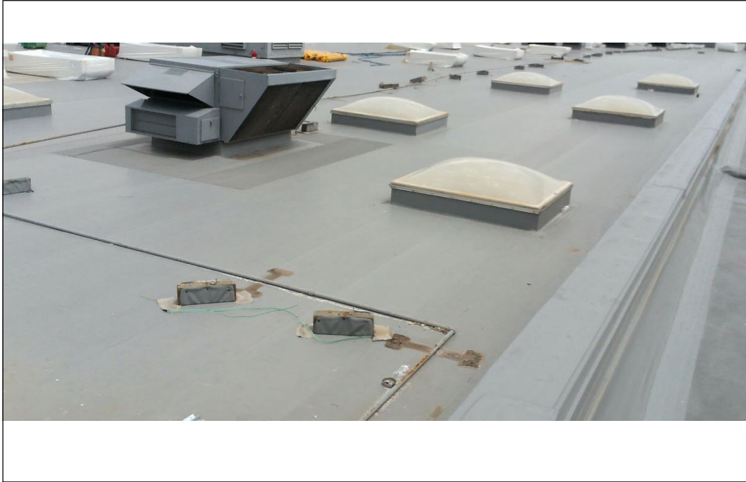
Fig. 3.1.1-3. Undamaged single-ply membrane roof cover adjacent to damaged roof in Figures 3.1.1-1 and 3.1.1-2
