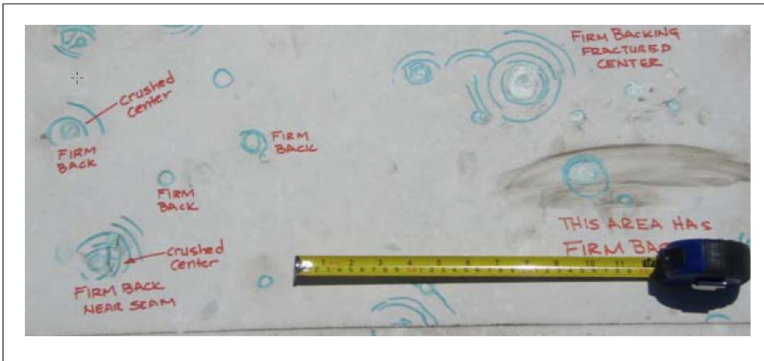
Fig. 3.5.2-2. Close-up of hail damage in Figure 3.5.2-1
