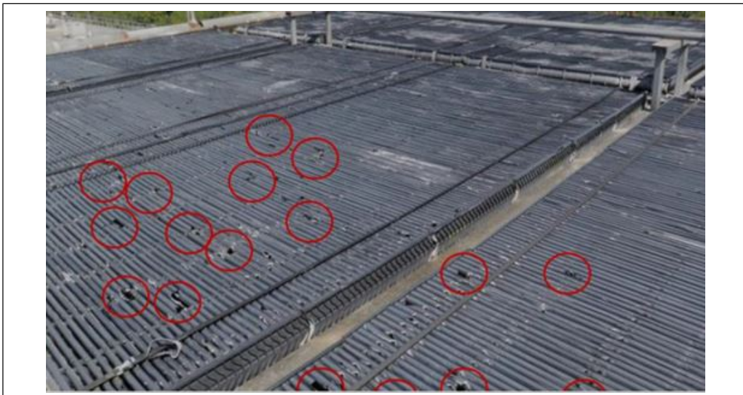
Fig. 3.4.1-2. Hail damage to plastic drift eliminators
