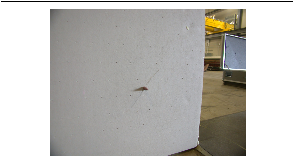
Fig. D.4.2.2-3. Crack in underside of cover board at fastener and beneath where crease was visible in the single-ply roof cover
