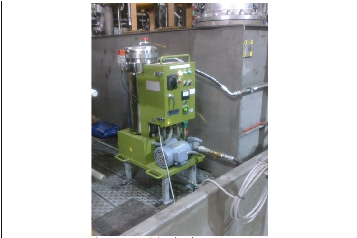
Fig. 4. Lube oil purifying skid inside containment area
