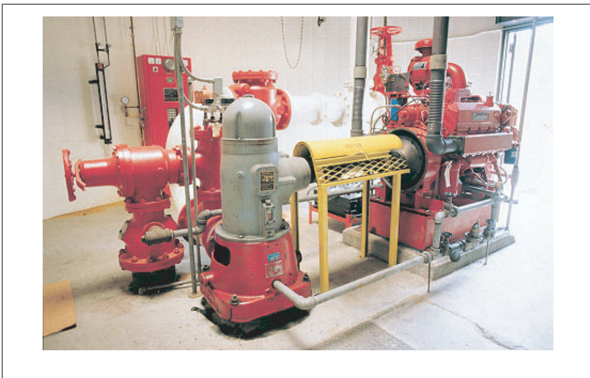
Fig. 2.2.1.2-1 Photo of well arranged pump room
